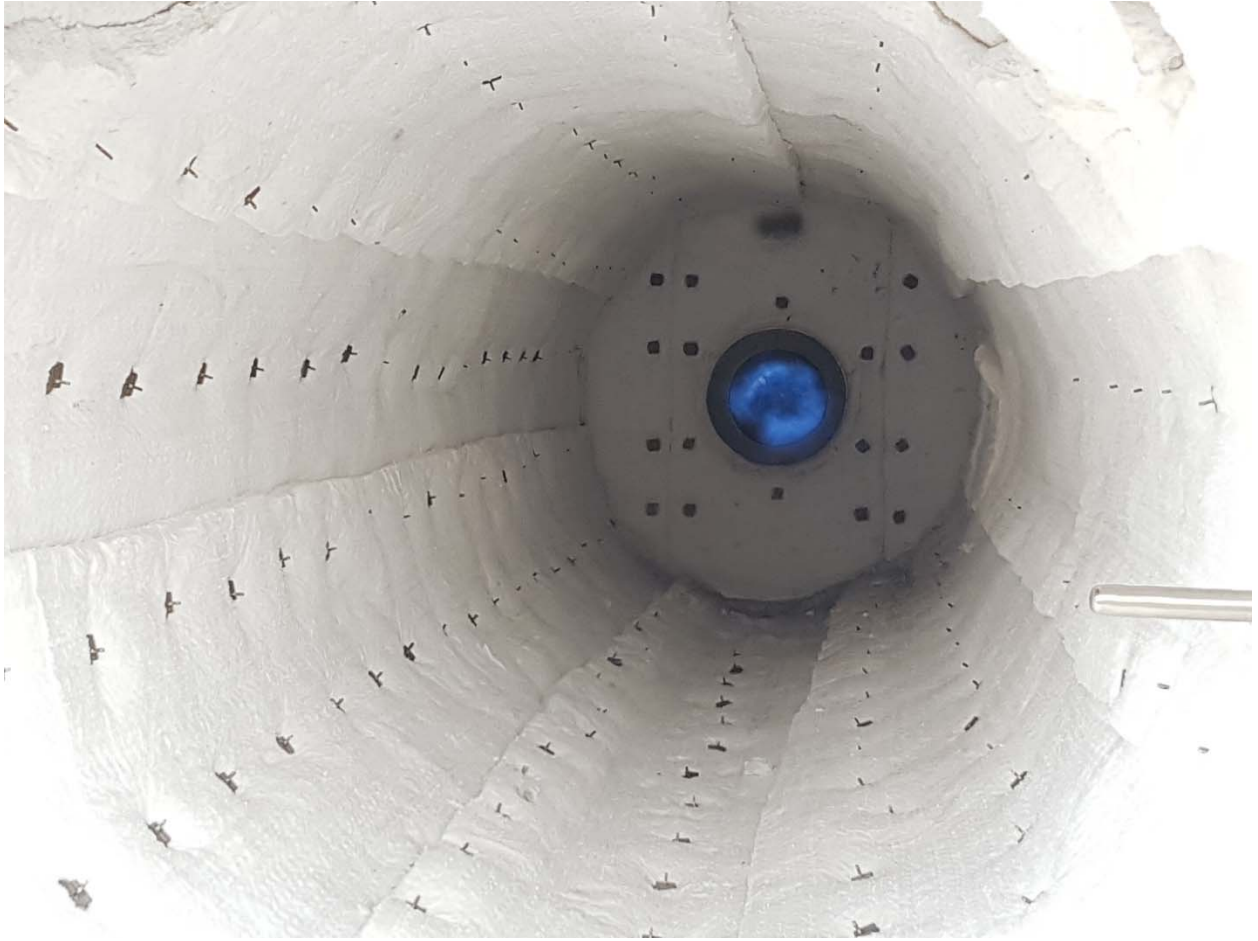
Fig 3: Example of High Temperature Morgan Thermal Ceramics Insulation with Long life Inconel Studs.
